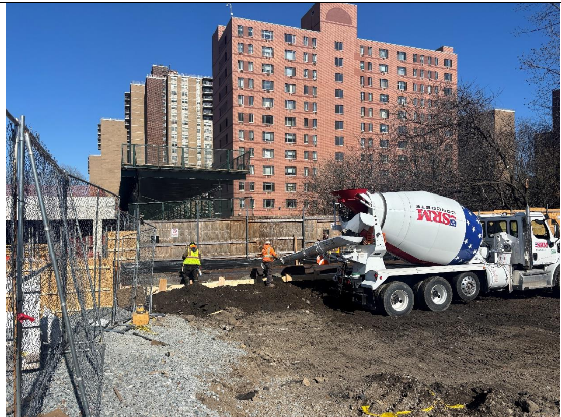
Photo 4 – RYC Turbos pouring concrete for the SOE guide wall in the southeastern portion of the Site, facing east.
