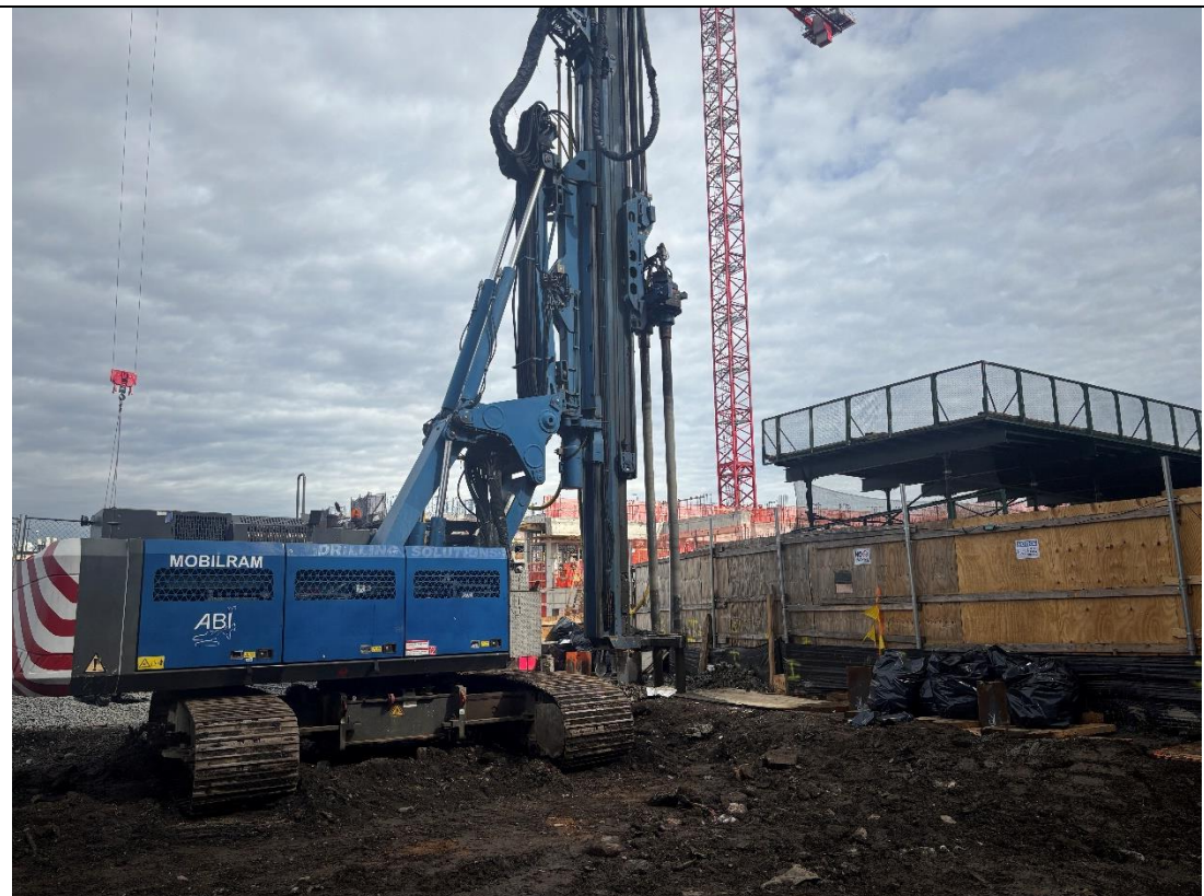
Photo 4 – RYC Turbos installing the soil mix wall in the southeastern portion of the Site, facing northeast.
