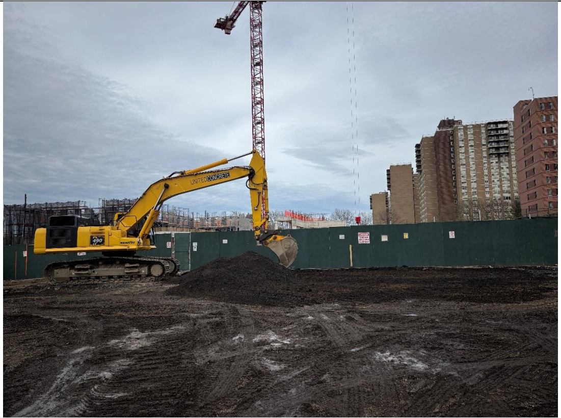
Photo 3 – United removing asphalt in the central portion of the Site, facing east.
