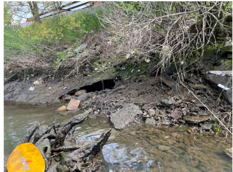
Photograph 4: Stormwater outfall and surrounding debris.
