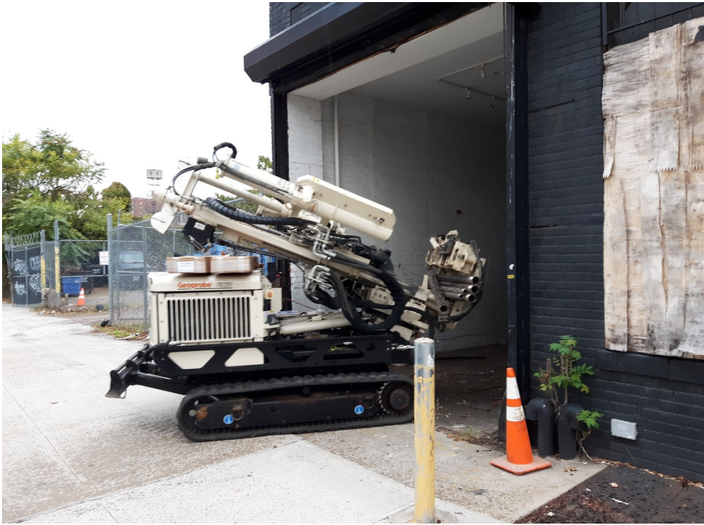
Photo 1: View of Geoprobe unit moving into 2-story building for install of MW-2.
