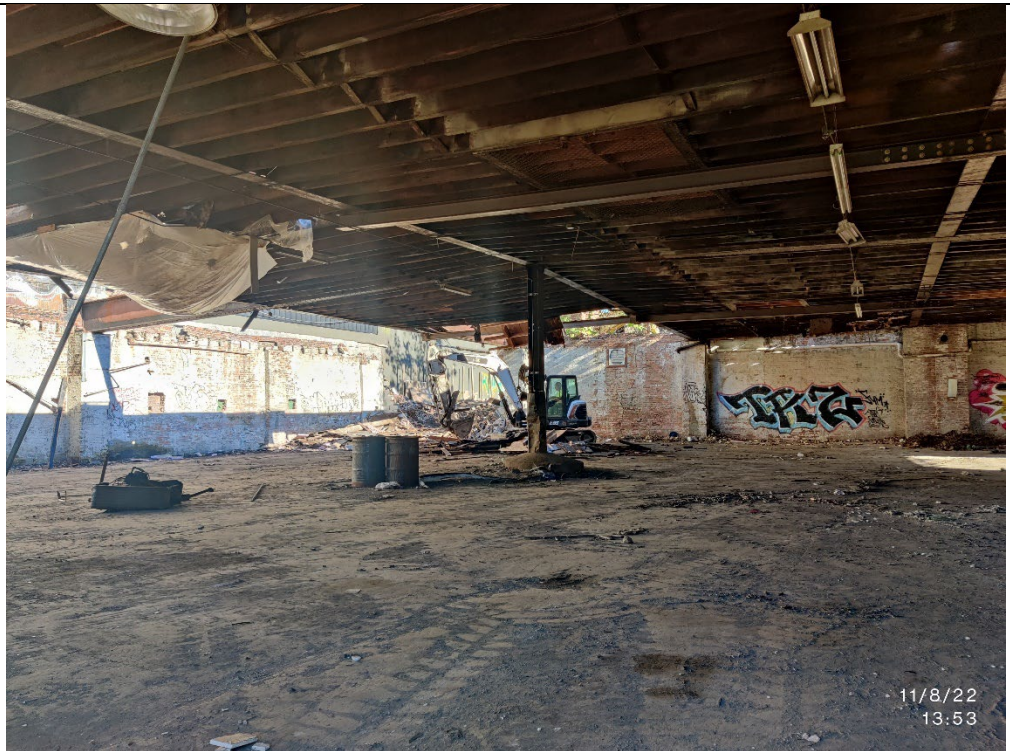
Photo 4 – Additional view of demolition in progress within the larger warehouse structure located on the western portion of the Site.
