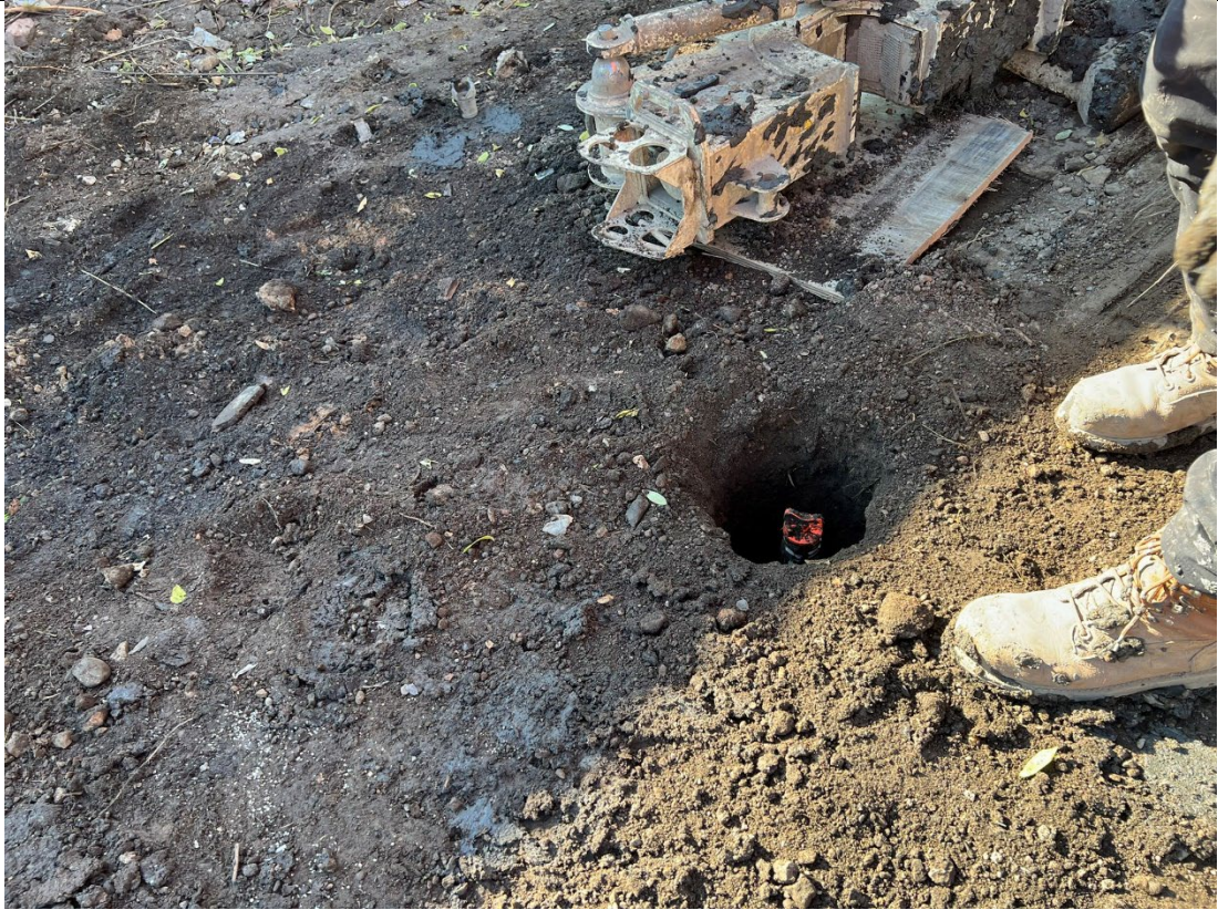
Photo 3 – Photo of shallow GW-8 well prior to installation of the manhole cover
