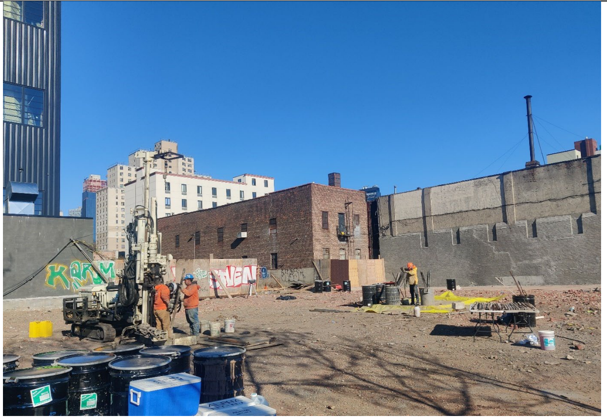
Photo 3- Representative photo of the Site at the end of the days activities.
