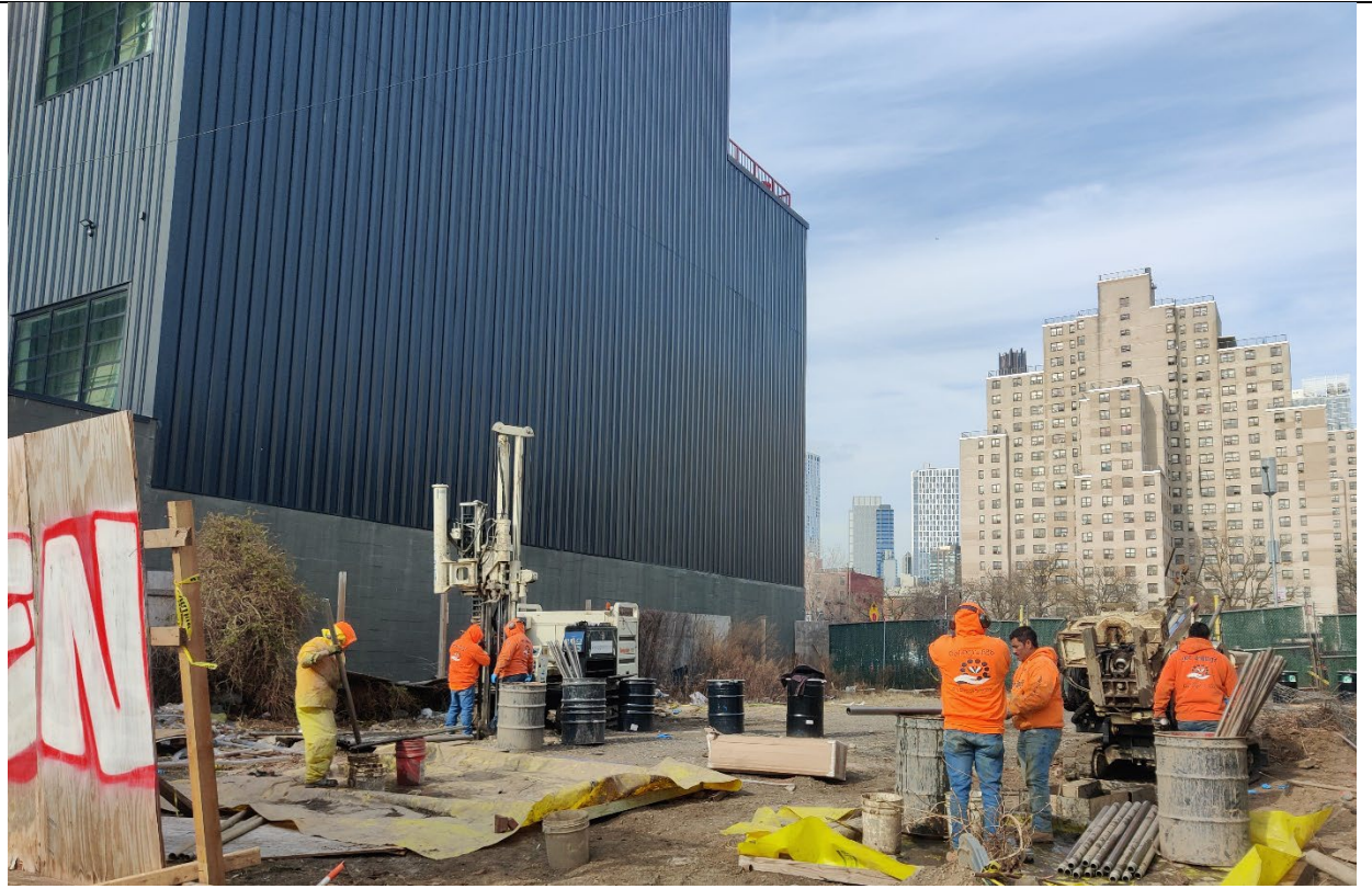
Photo 3- Representative view of the Site at the end of the day's activities.
