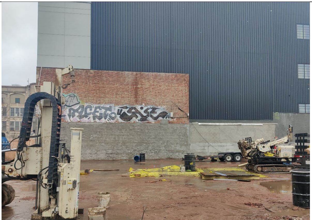
Photo 4- Representative view of the Site at the end of the day's activities. Borings, DB-33(right) and DB-30 (left).
