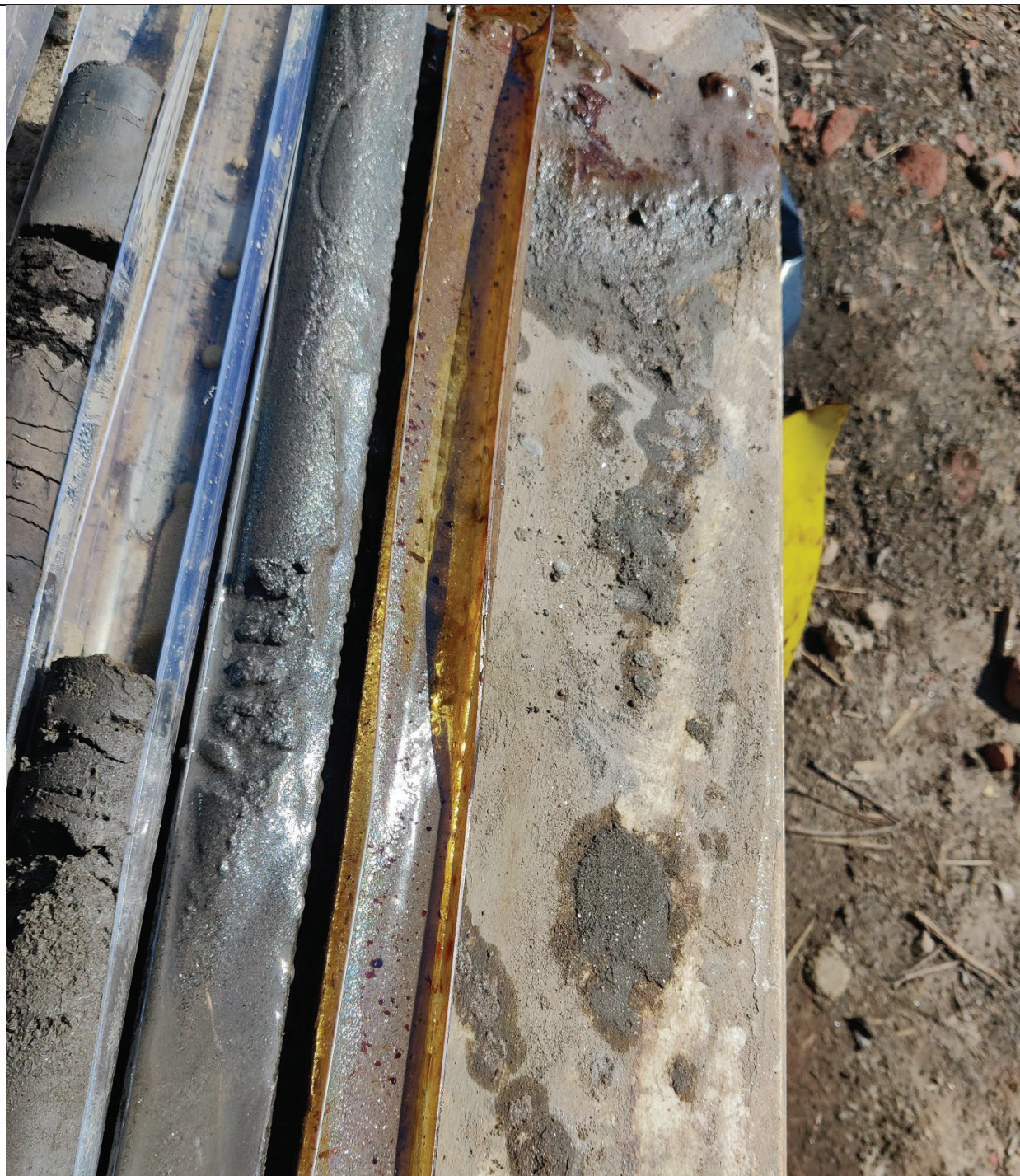
Photo 2- View of boring DB- 13, with MGP coal tar blebs at the 35-37' interval
