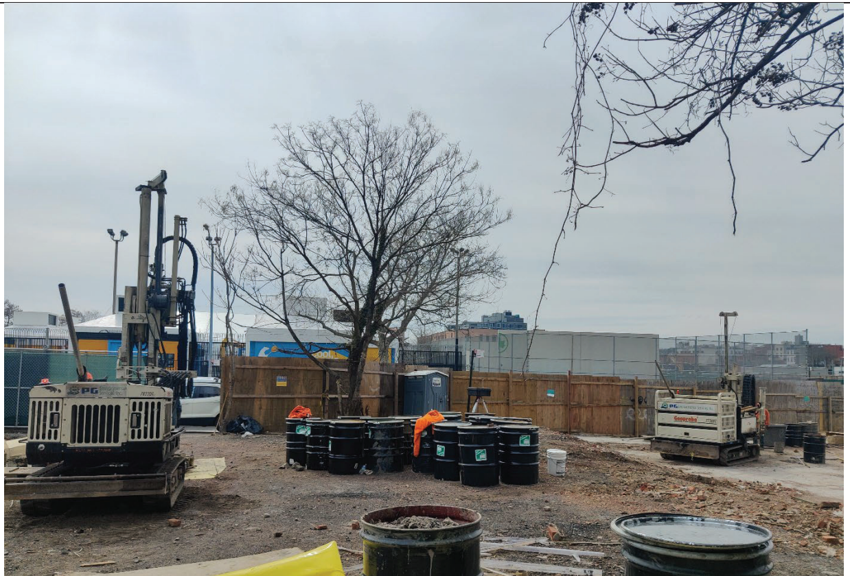
Photo 4- Representative view of the Site at the end of the day's activities. Borings DB-3 (left) and DB-31 (right).
