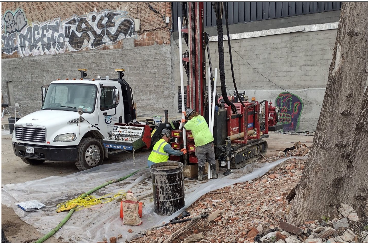
Photo 2- Representative view of installation of CW-4-85, Coastal utilizing mud pan in order to contain liquid coming off tooling when pulled out.
