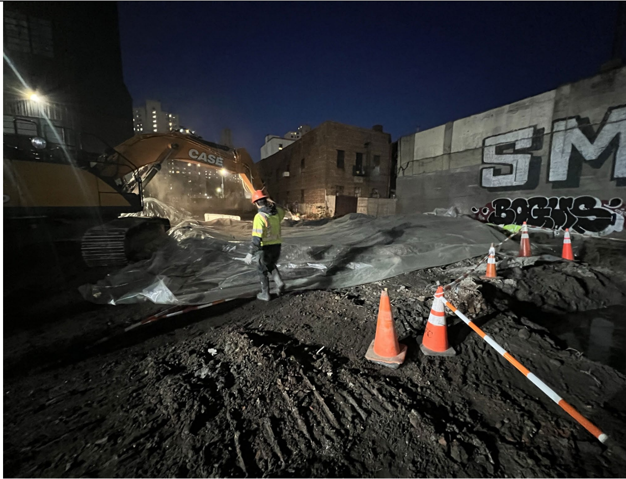
Photo 5- Representative photo of all material covered with poly at the end of the day
