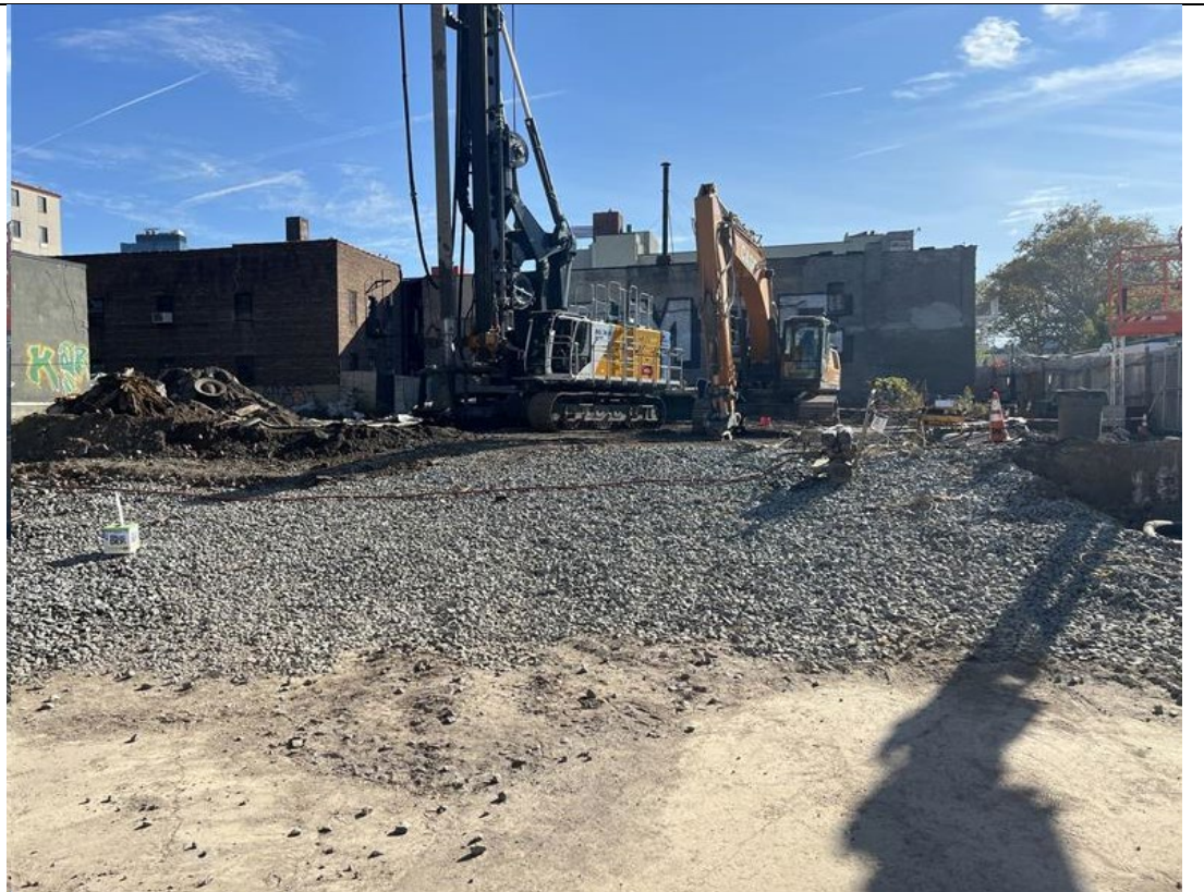
Photo 2 – Cascade rig at top of ramp where treatment columns were relocated to column 304.
