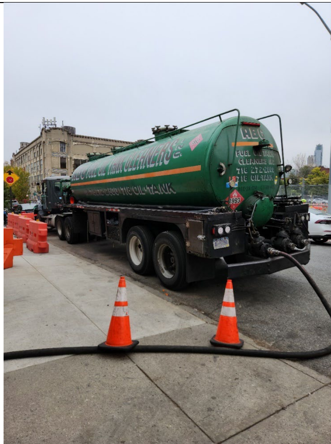
Photo 4 – Representative view of the pump truck used to remove the liquid from the unregistered 550-gallon tank.
