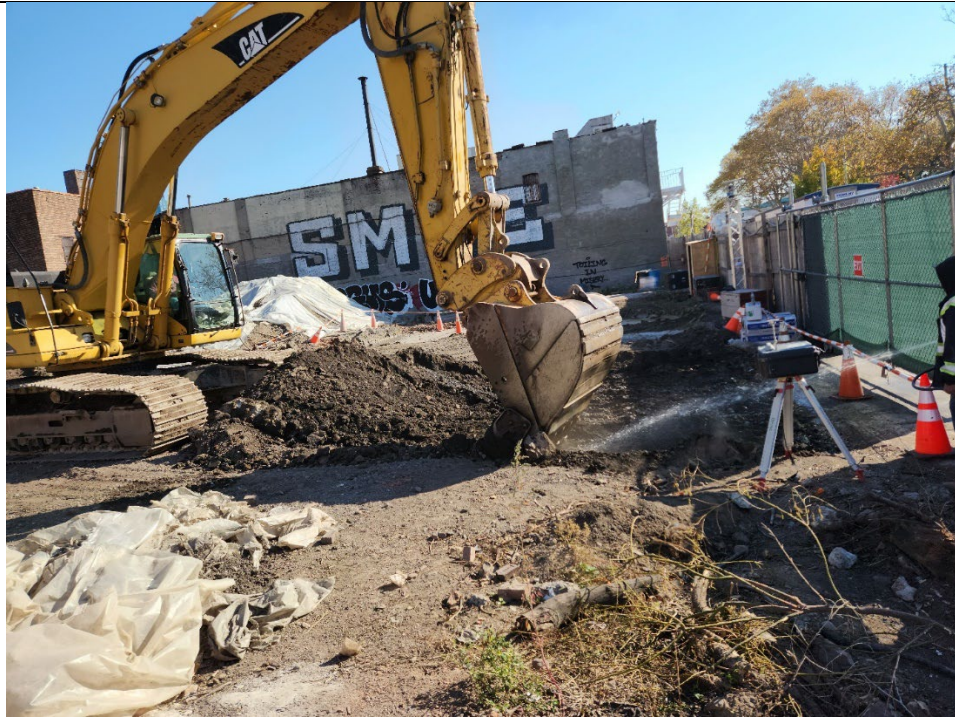
Photo 3 – Representative photo of active water suppression at truck entrance along Douglass Street where stone was being added.
