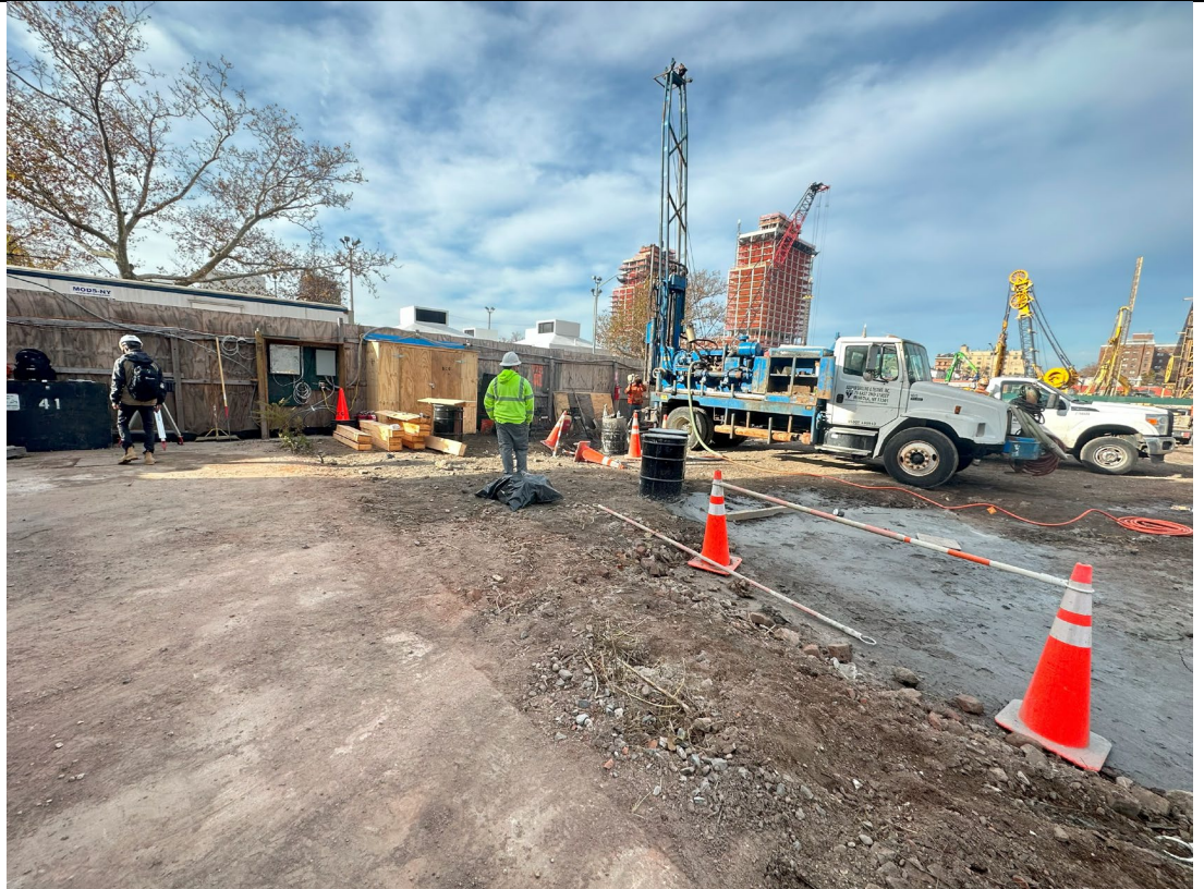
Photo 2 – Representative view of the southeast side of the Site where drilling is getting done (Mix C- Column 25).
