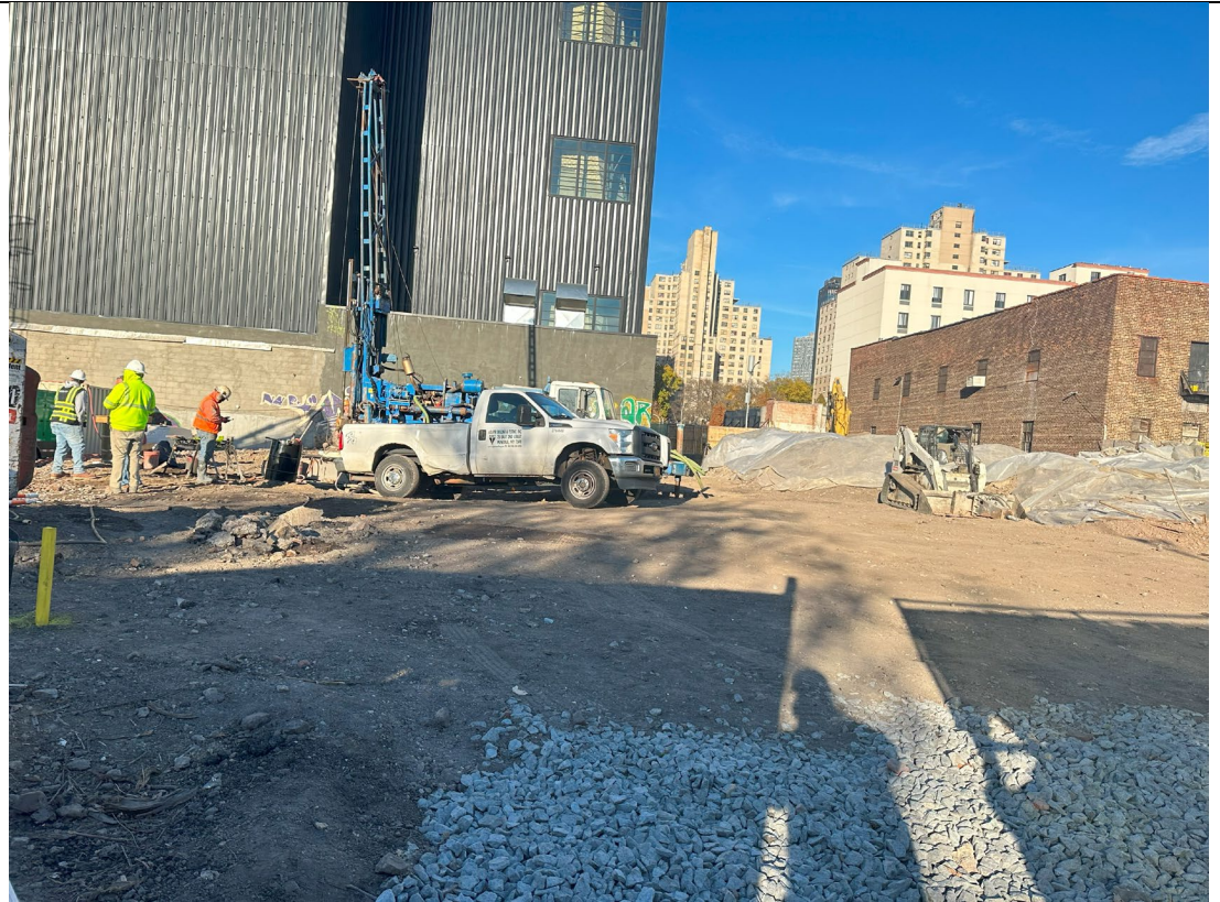
Photo 1- Representative phot of the north side of Site, ADT coring at the overlap of Columns 304 and 337.
