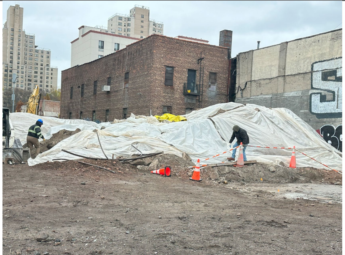
Photo 4 – Representative view of BCG Laborers covering stockpiles securely with poly in preparation for heavy rain.
