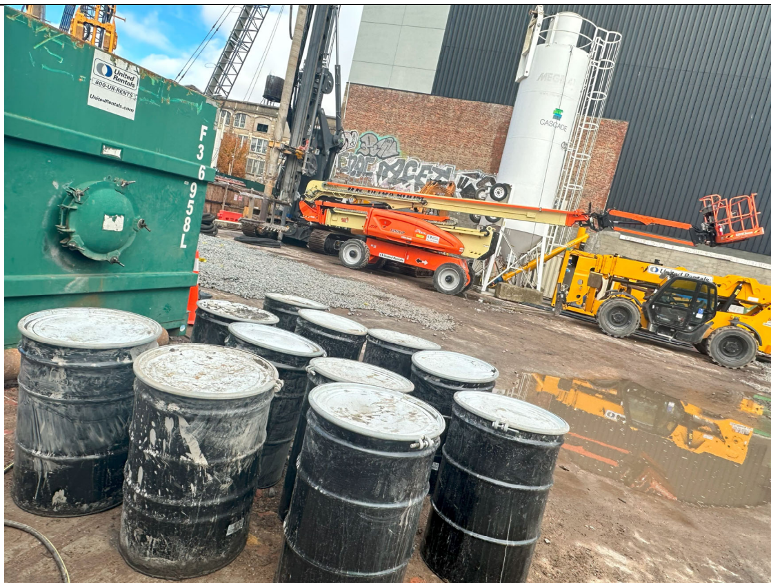
Photo 4 – . Generated 11 drums in total containing decon water from core drilling pilot test columns.
