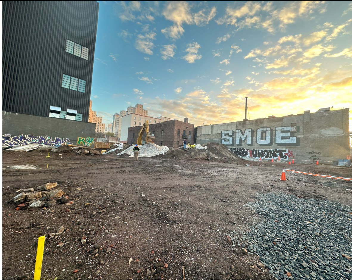
Photo 1- Representative view of the site prior to truck loading. Removal of plastic cover from stockpiled ISS spoils.
