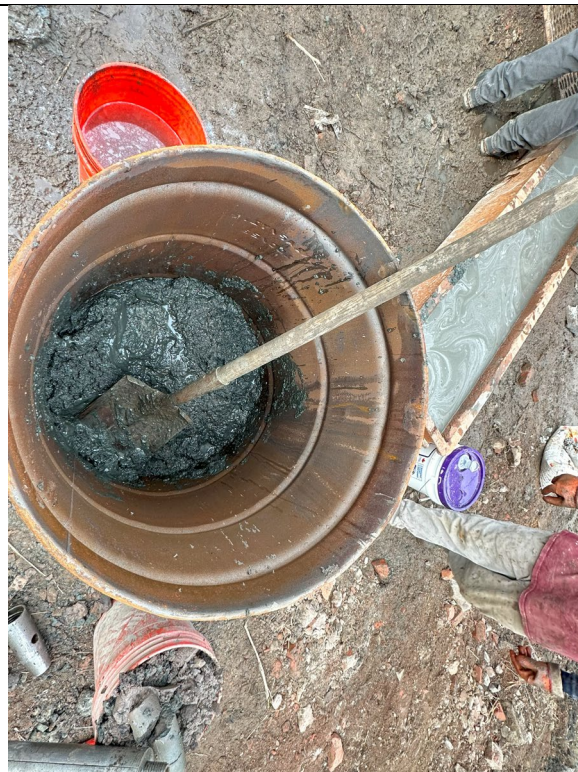
Photo 2 – Representative photo of GES storing excess dirt from boring and mug pan water into drums. This material is being separated from each mix type.
