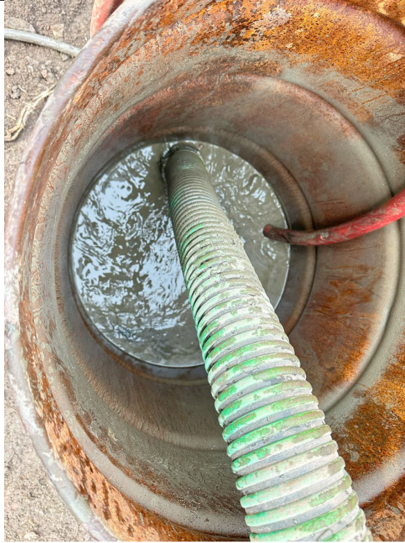
Photo 3- Representative Photo grout being used to fill boring hole at Mix A (Columns 154, 155 and 102).
