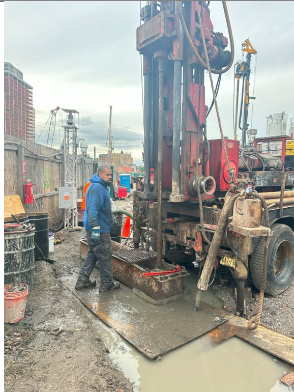
Photo 4 – Representative photo of grout being used to fill boring hole to grade at Mix C location.
