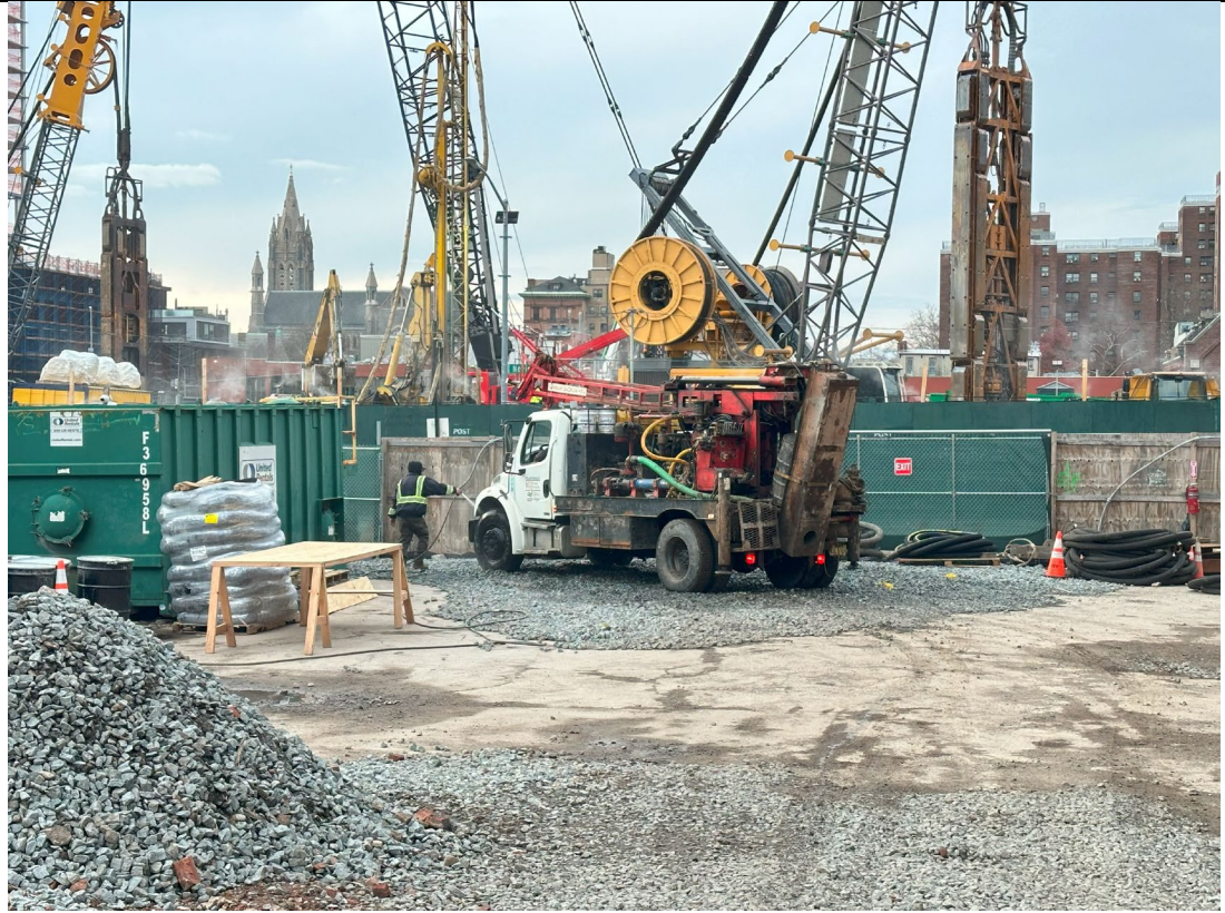
Photo 5- Representative view of GES rig tires being washed at truck wash prior to leaving the Site.
