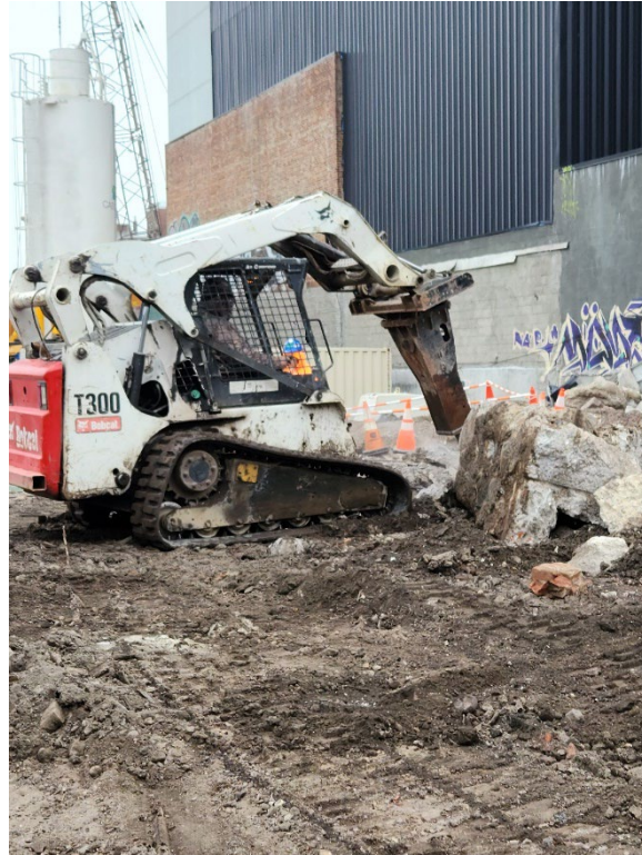
Photo 1- Representative view of skid steer breaking apart concrete into smaller pieces for offsite disposal.
