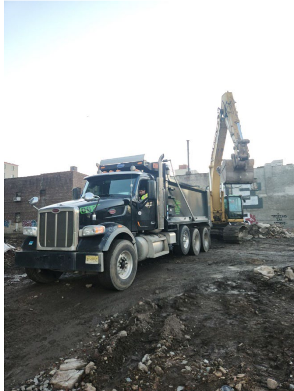
Photo 1- Representative view of truck being loaded with concrete for disposal to PPark.
