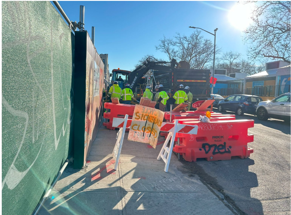
Photo 2 – Representative view of National Grid working offsite on sidewalk adjacent to Douglass Street.
