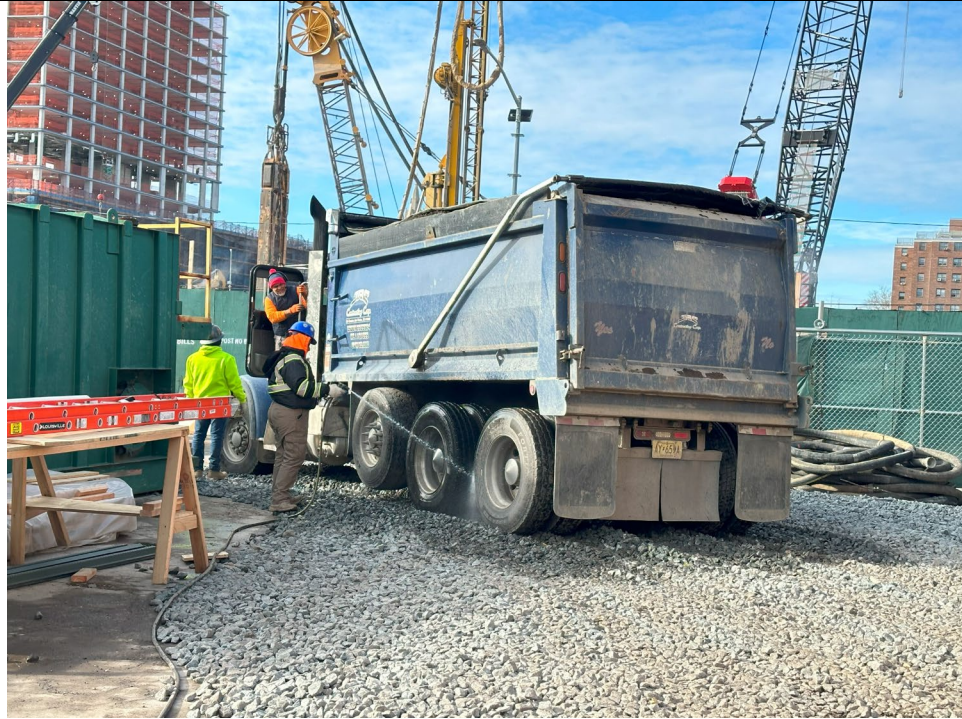
Photo 2 – Representative view of truck tires being washed off on the truck pad/ decon area.
