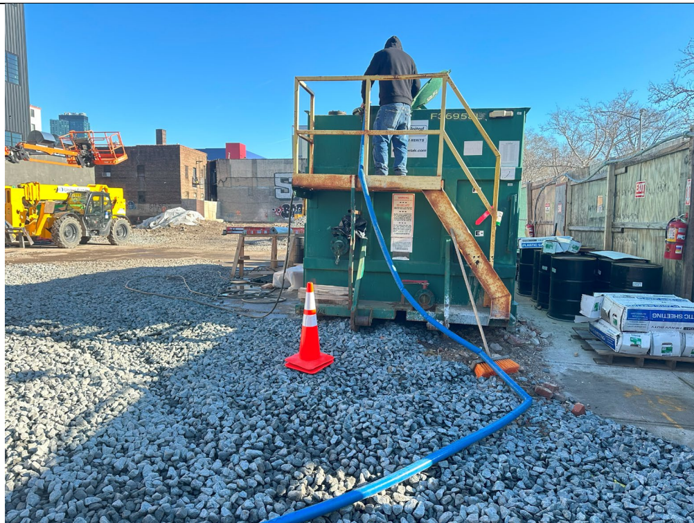
Photo 4- Representative view of truck wash holding tank being pumped into frac tank in preparation of heavy rain event.
