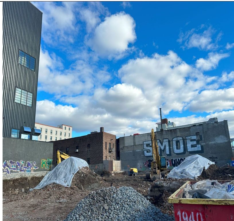
Photo 4- Representative view of material stockpiles covered with poly sheeting at the end of the days activities.
