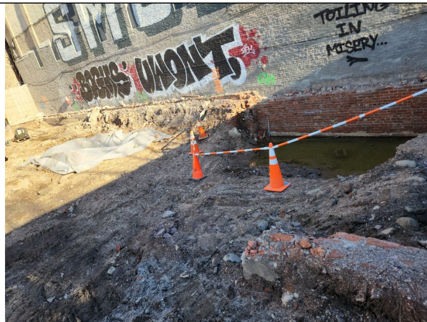
Photo 4- Representative photo of tank grave covered with poly.
