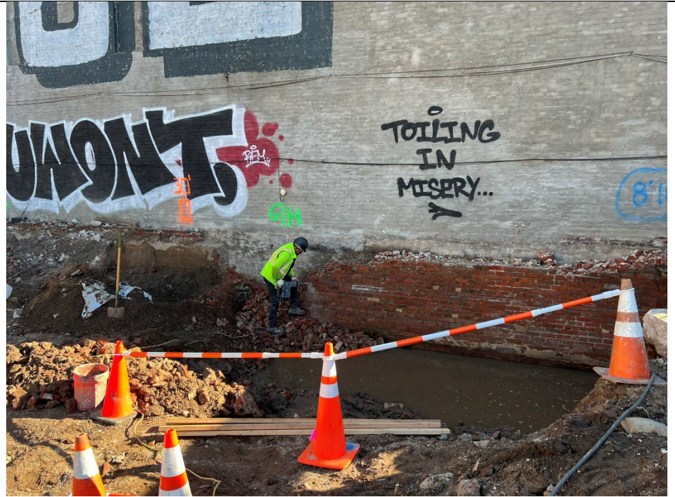
Photo 1- Representative view of hand demolition work on the western portion of the Site.
