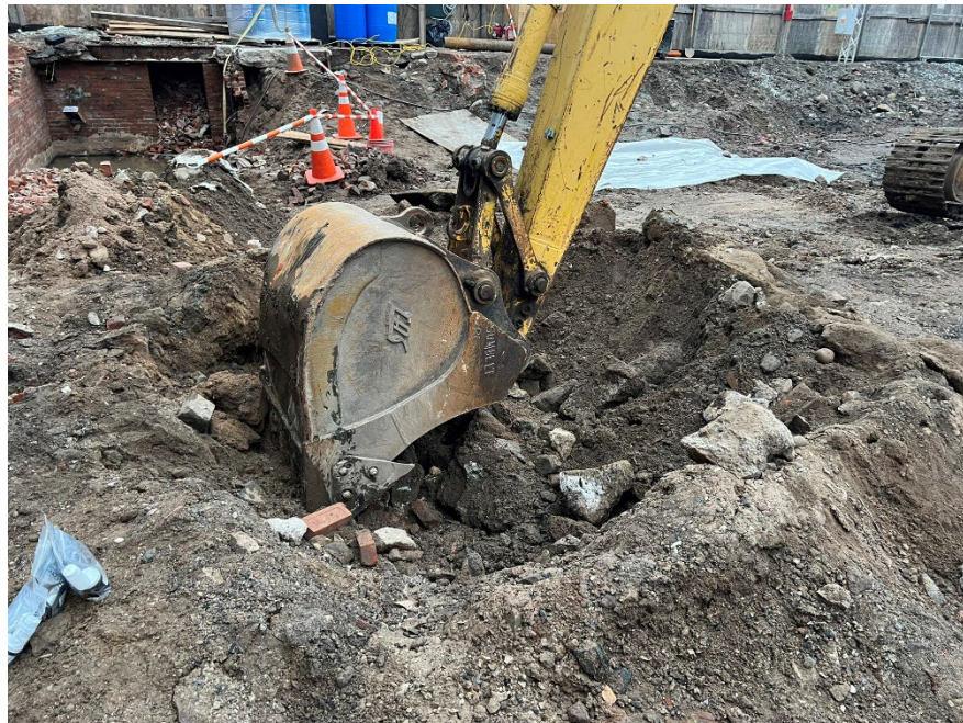
Photo 2 - Representative view of over excavation of Tank-2.
