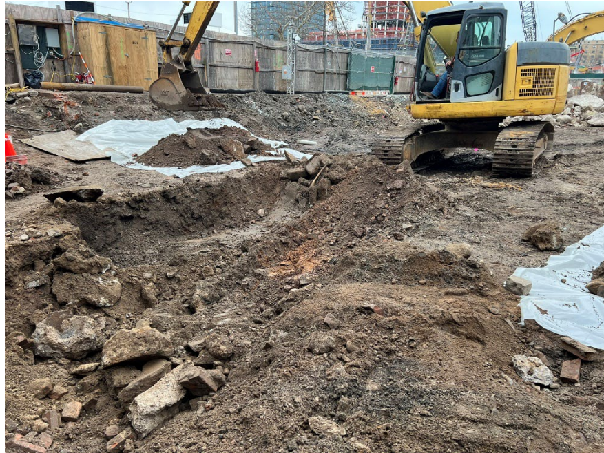
Photo 1 – Representative view of excavation of the arsenic hot spot, excavated material placed on poly.
