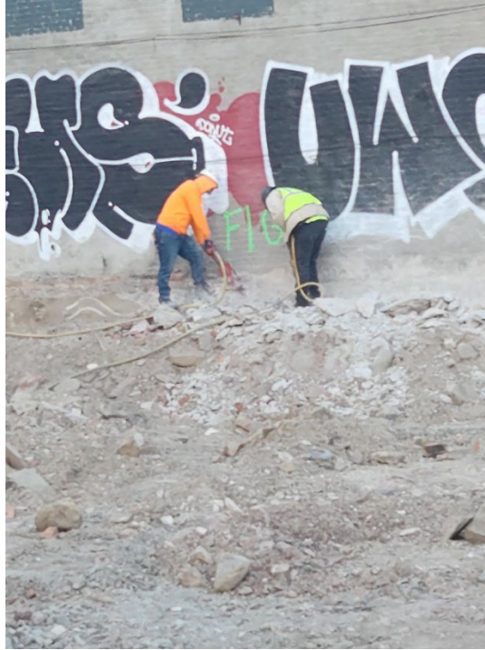
Photo 1 – Representative view hand demolition/ chipping of concrete from old building on eastern portion of the Site.
