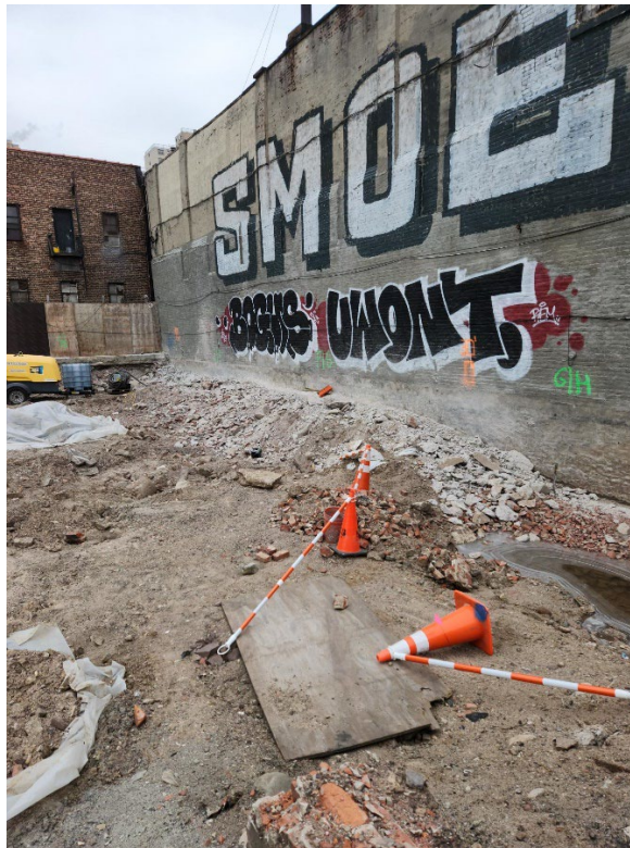
Photo 2 – Representative view looking north of the eastern portion of the Site post demolition of concrete wall.
