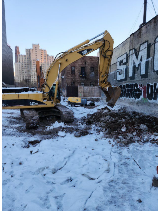
Photo 1 – Representative photo of the excavator clearing the area proximal to the east wall.
