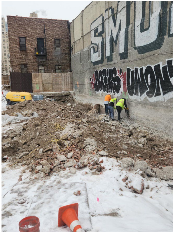
Photo 2 – Additional representative view of Xolle crew performing hand demolition along east concrete wall.
