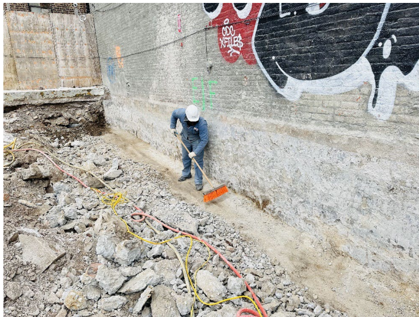
Photo 2 – Additional view of Xolle crew working along eastern portion of the Site.
