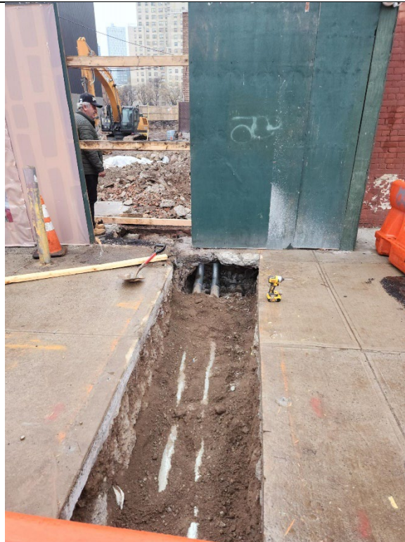
Photo 2 – Representative view of electrical piping Con Ed was accessing off-site.
