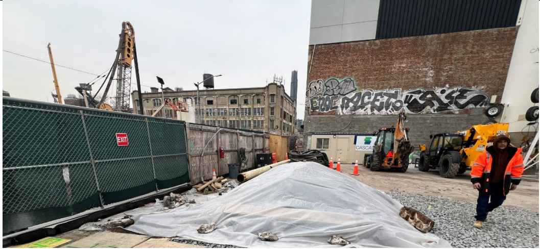
Photo 1- Representative view of material from the sewer connection work placed on top of and covered with poly for sampling and disposal.
