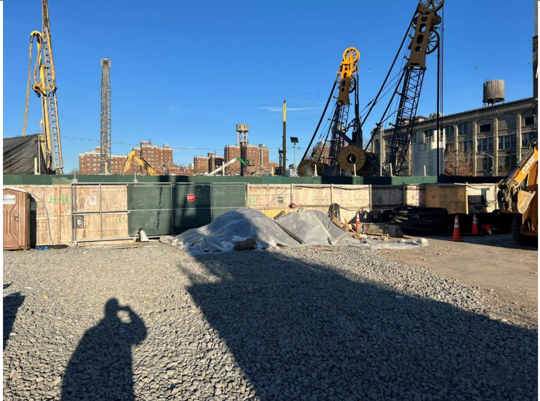
Photo 1- Representative view of material excavated during the sewer connection staged and covered with poly.
