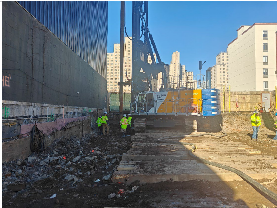
Photo 4- Cascade tests Bauer rig in preparation to begin ISS columns in the northwest corner of the Site along Butler Street beginning 2/20/24.
