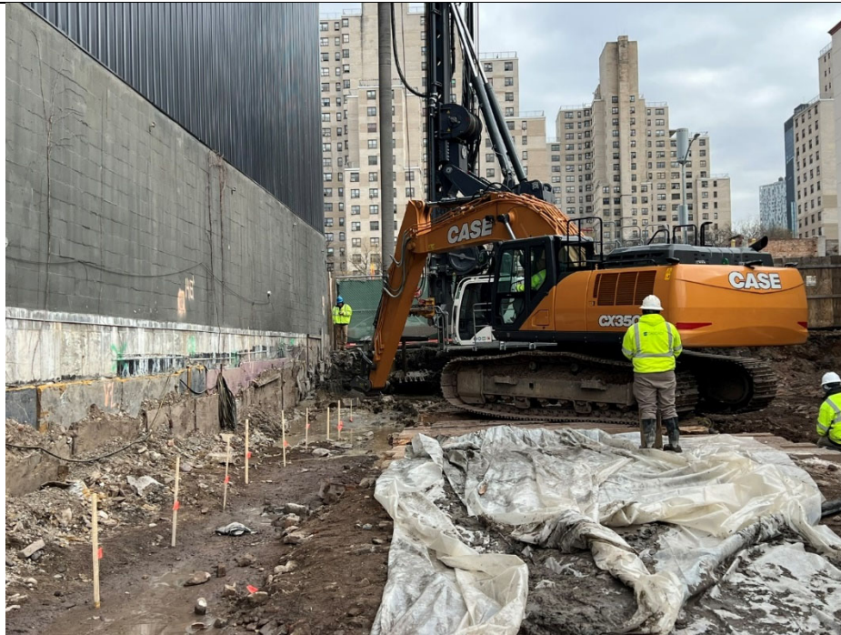
Photo 4- Representative photo of attempting to remove an obstruction.
