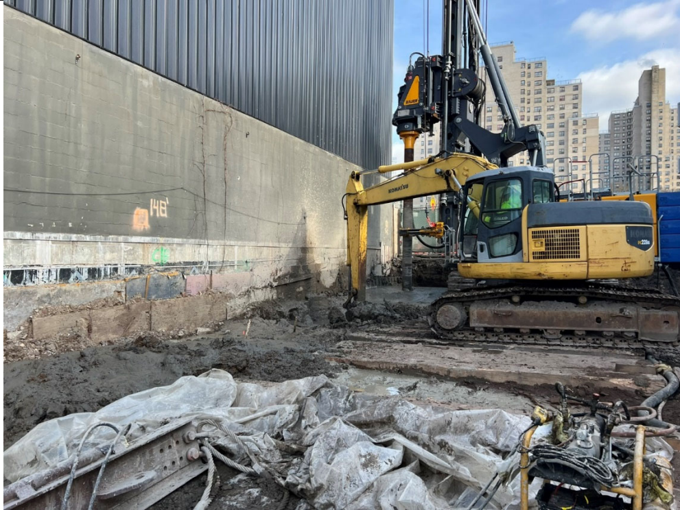
Photo 1- Representative photo of attempting to remove the obstructions from 2/21/2024.
