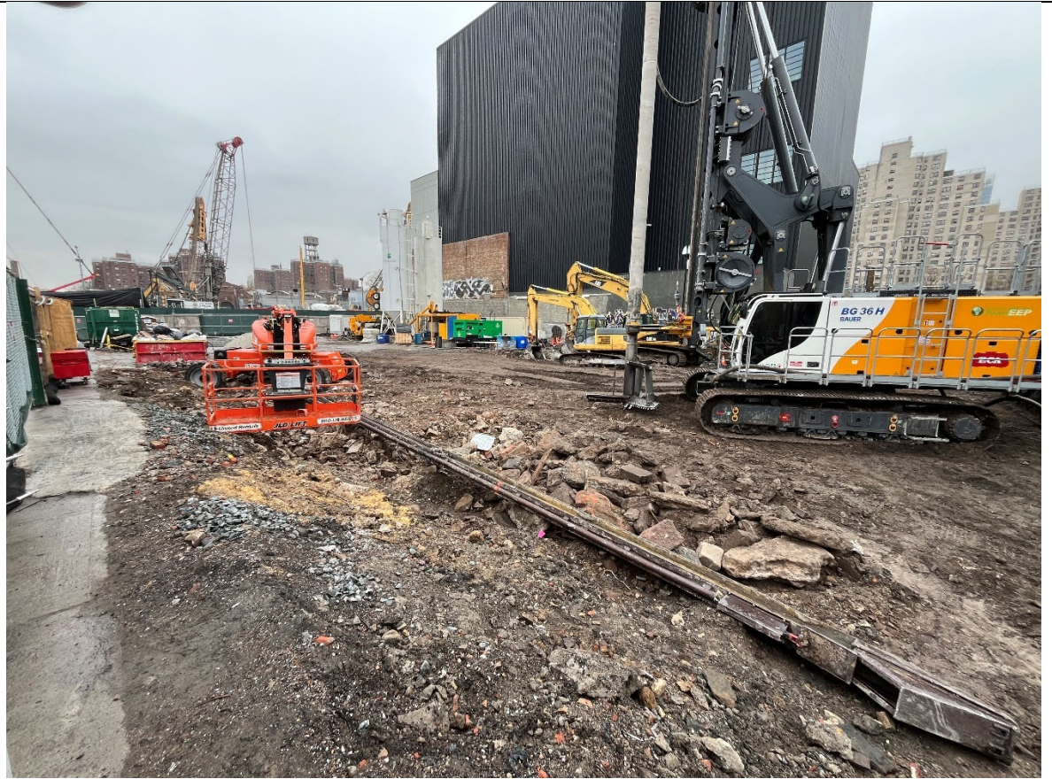
Photo 5- Representative photo of the southern portion of the site at the end of day.
