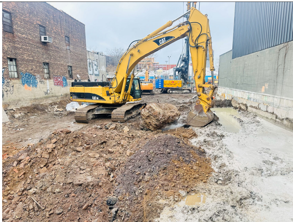
Photo 2 – Representative photo of concrete obstruction.
