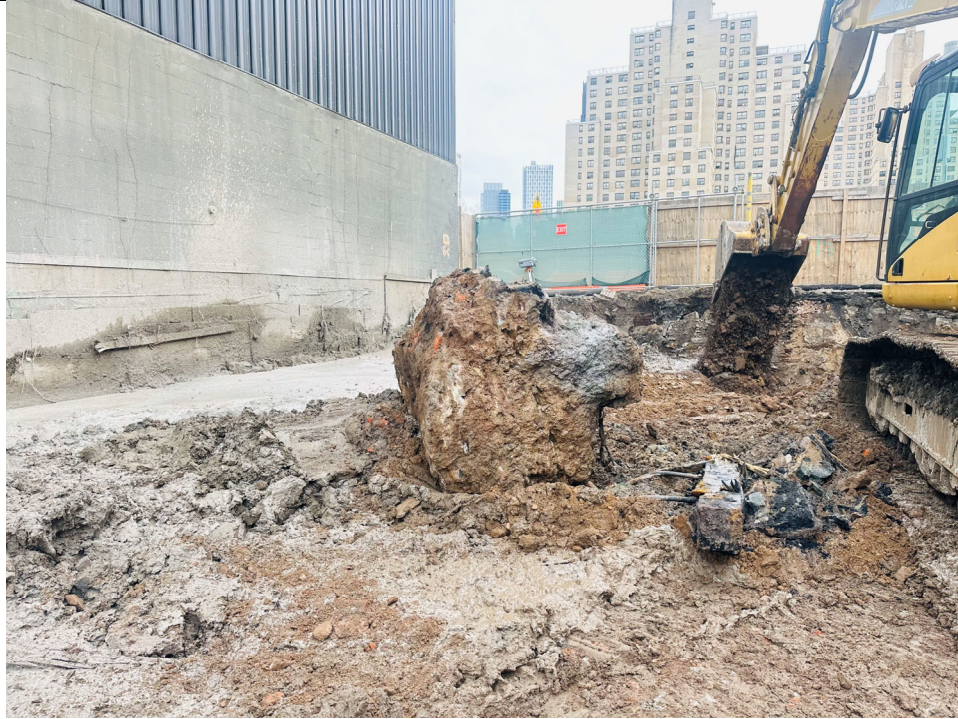
Photo 3- Representative photo of concrete obstruction.
