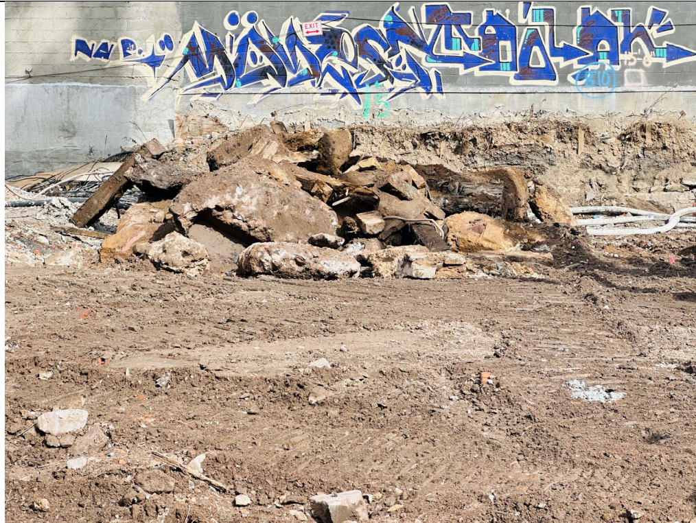
Photo 5- Representative photo of concrete obstructions removed at the end of the days activities.
