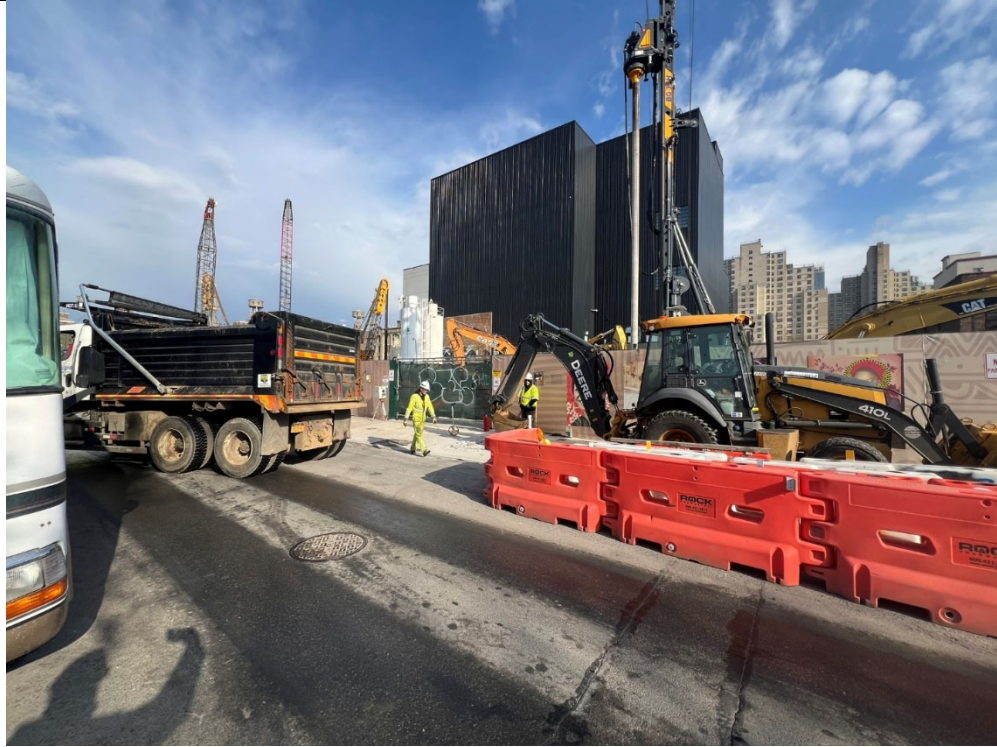
Photo 3- Representative photo of national grid working in the sidewalk on Douglass Street.
