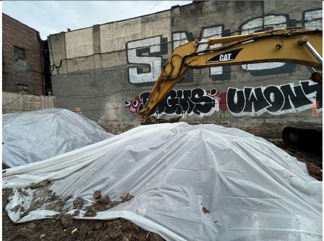
Photo 5- Representative photo of stockpiled material covered at the end of the workday.
