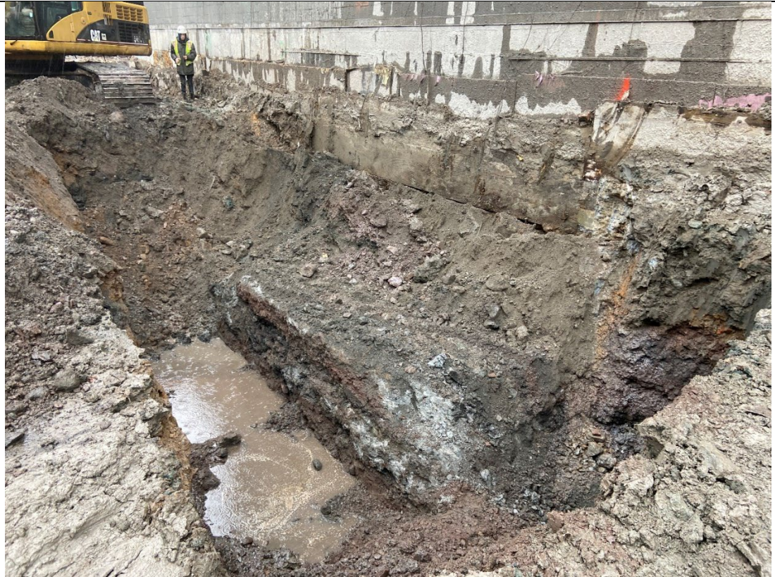
Photo 3- Representative photo of concrete slab found on excavated area, obstruction measures 20' long x 9' wide and 3 feet deep.
