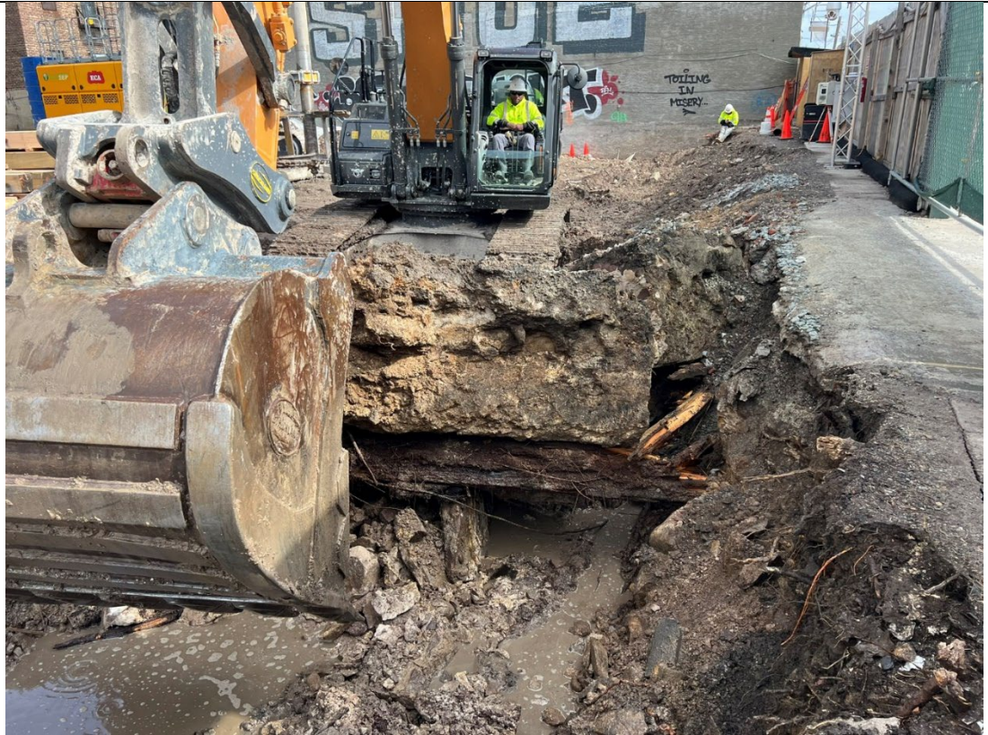
Photo 3- Representative photo of obstructions being removed on the southern portion of the site adjacent to Douglass Street.
