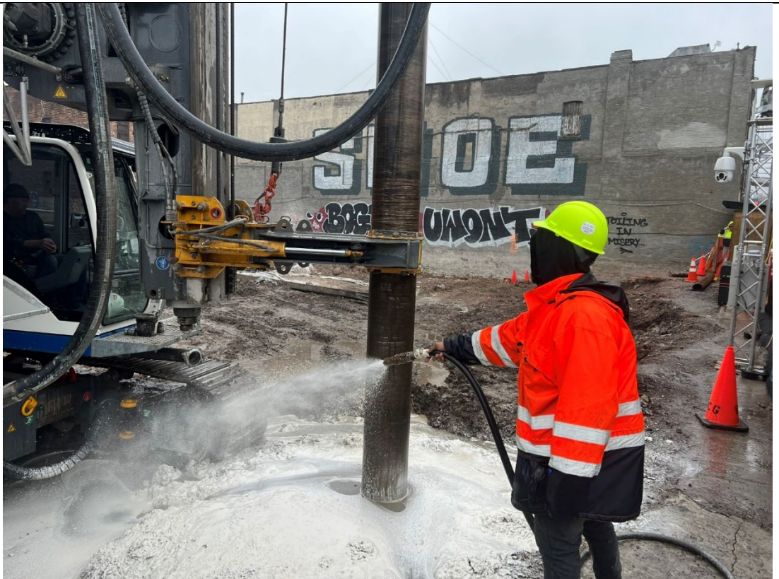
Photo 2- Representative photo of ATMOS foam being sprayed while drilling an ISS column.
